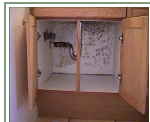
Common places for mold growth include storage space underneath sinks.
