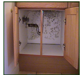
Common places for mold growth are cabinets under sinks, often due to pipe leaks.
